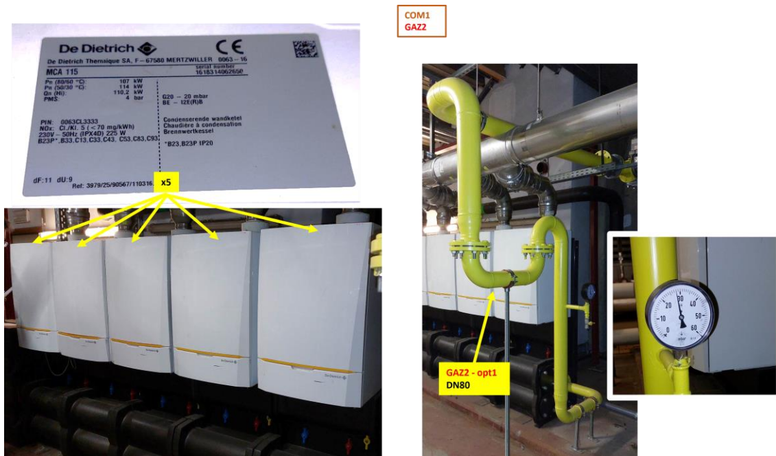
Figure 26: Pictures and description of the Brussels LL boiler room on the 4th Floor
