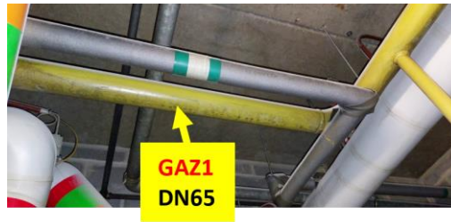
Figure 25: Pictures and description of the Brussels LL boiler room on -1 Floor
