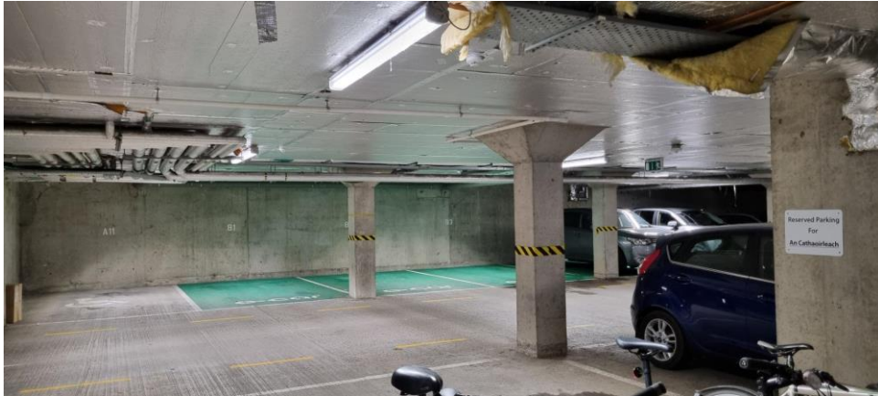
Figure 6: County Hall Basement - Battery Bank
